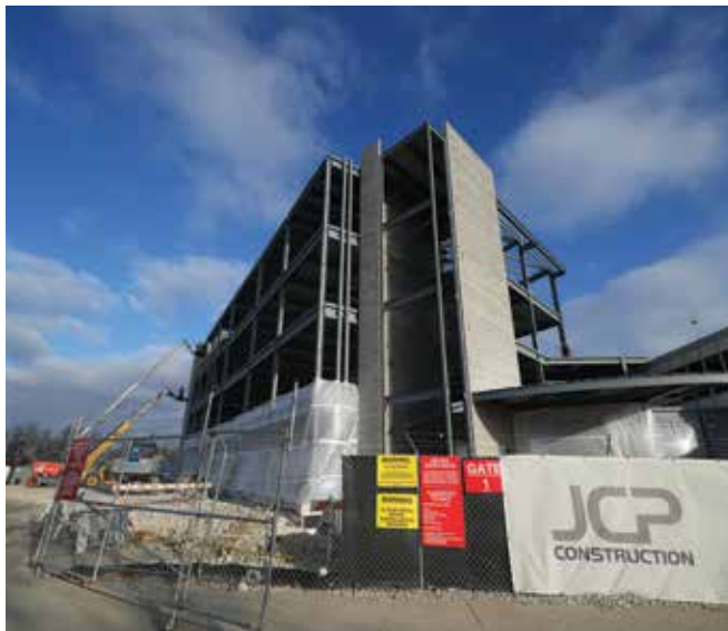
Outreach Community Health Center's new Capitol Drive clinic under construction in 2023. JCP, one of the Foundation's impact investing loan recipients, was the general contractor on the project.
